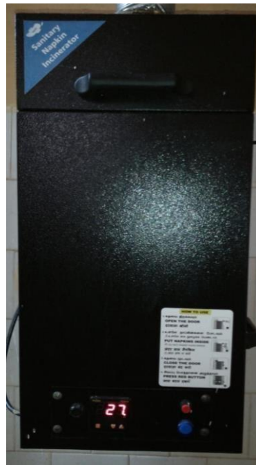
Napkin Incinerator Facility in the Girls' Rest room
