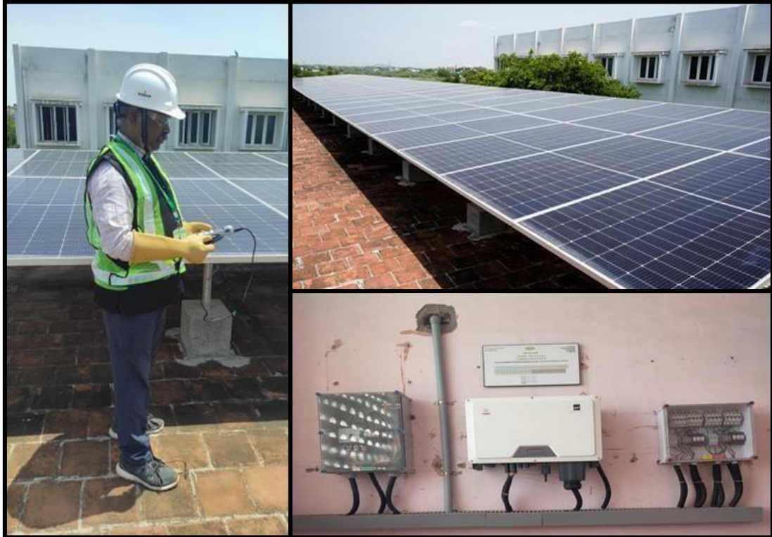
Solar Unit Panels Facility Available in the Mannar Thirumalai Naicker College, Madurai, Tamil Nadu
